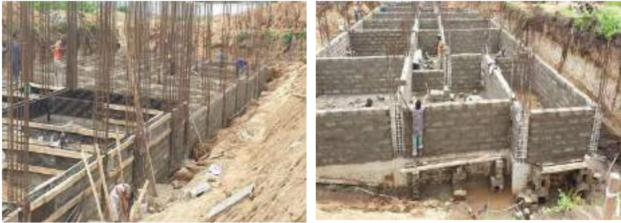
Figure 17: Still fixing and formworks for tie beams (left) and second round of foundation wall
